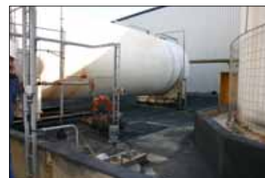
Linings in secondary containment
